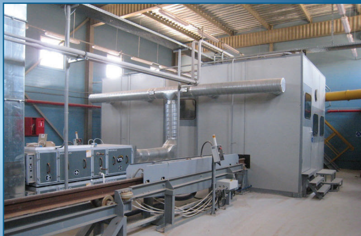
Final grinding station ПЧШ-01
